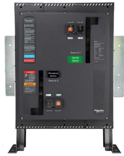
Transfer Switch Unit
